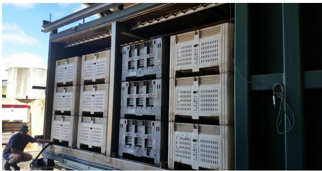
Hydro-vacuum cooler loaded with broccoli bins
